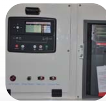
Control Panel & MCB
